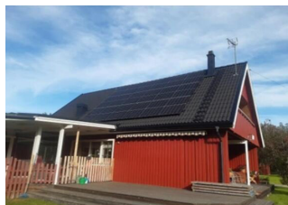
14.76KW in Sweden
